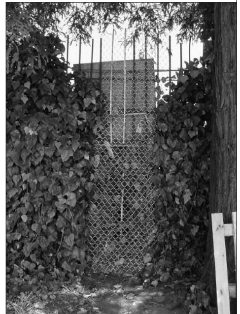
Fence with mission vertical posts and wire mesh after temporary repairs completed.
